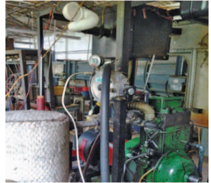
Inlet manifold assembled to diesel engine.
